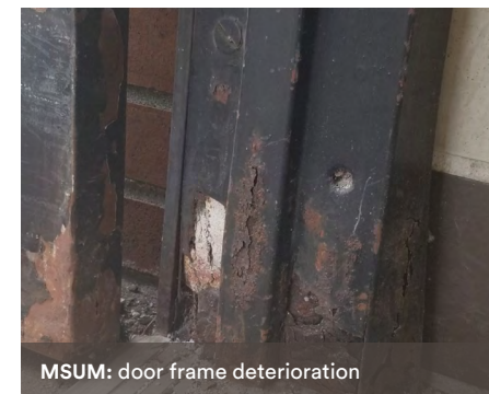
LSC: roof deterioration
