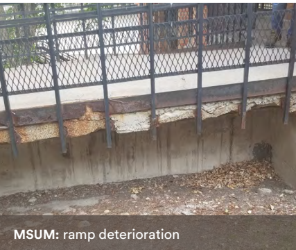
MSUM: concrete deterioration
